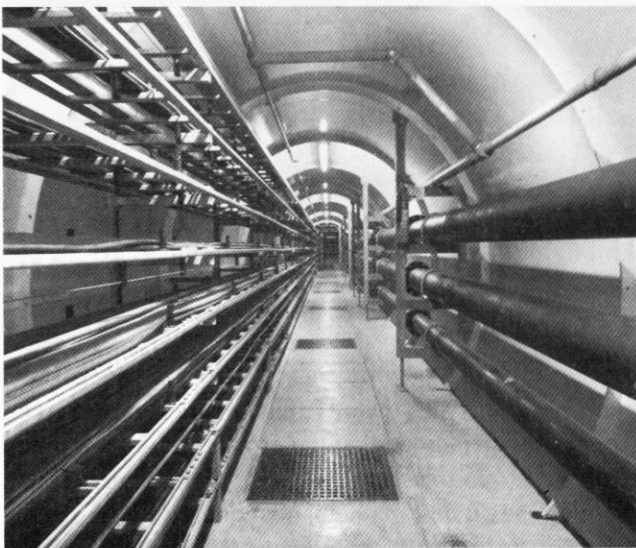
A typical view within a tunnel looking south – welded steel tube embedded in the precast concrete sill, power and comms cables to left; sprinkler, fire hydrant and water mains to right. The end of the tunnel in Pier 9 in the distance.
